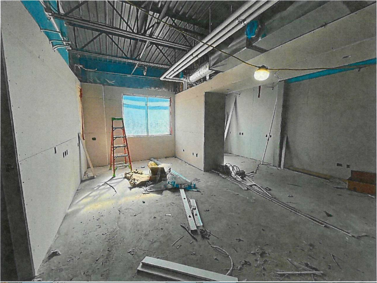
Most interior walls are framed, mechanical electrical and plumbing is roughed-in, and drywall is hung.
