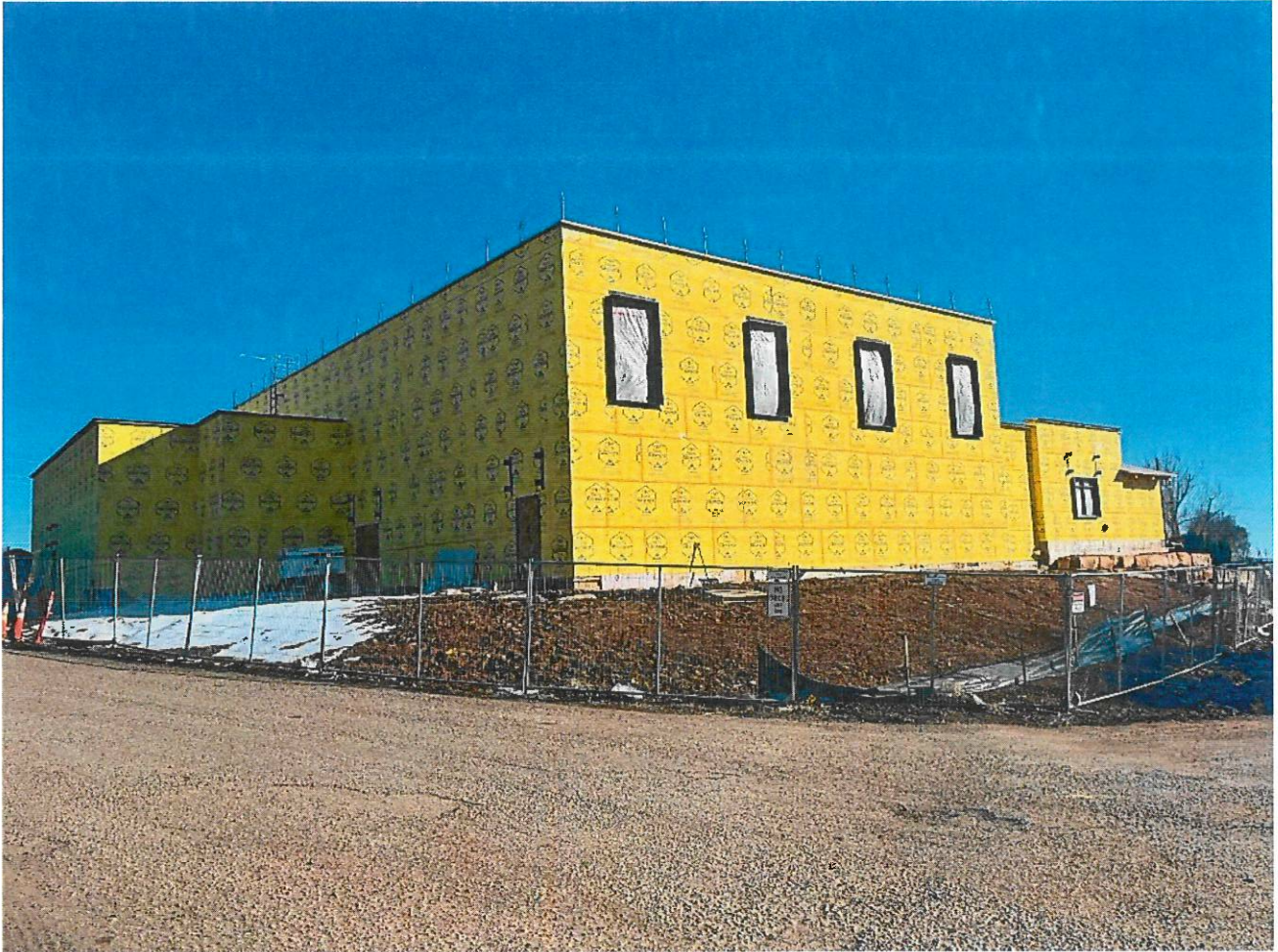
Exterior sheathing is nearly complete, window frames installed, roof installation ongoing. Window canopies and glazing to be installed soon.
