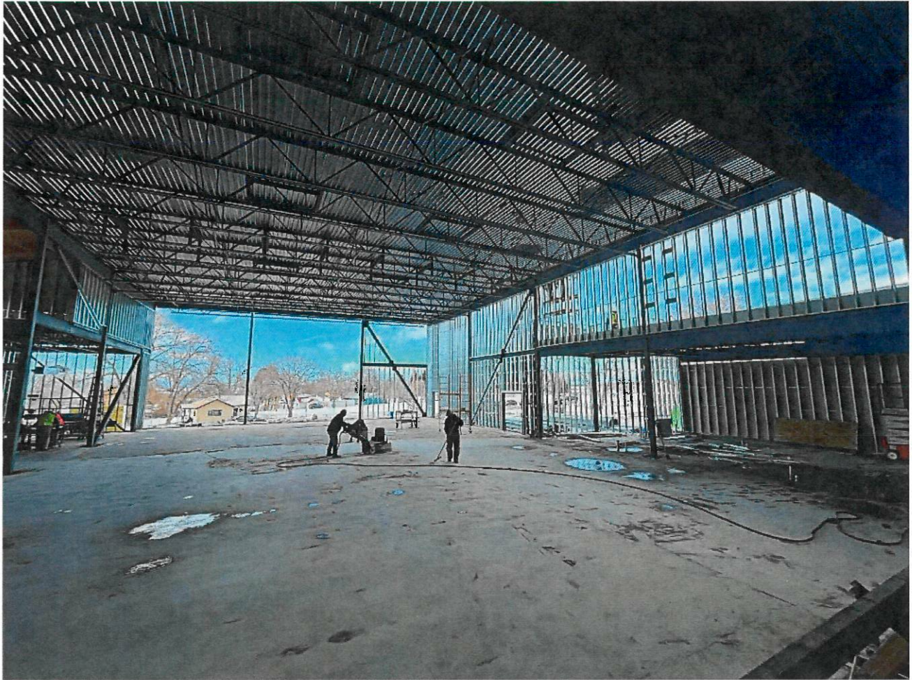
Floor grinding operations in the gym to achieve specified flatness and levelness. Exterior walls getting framed in.
