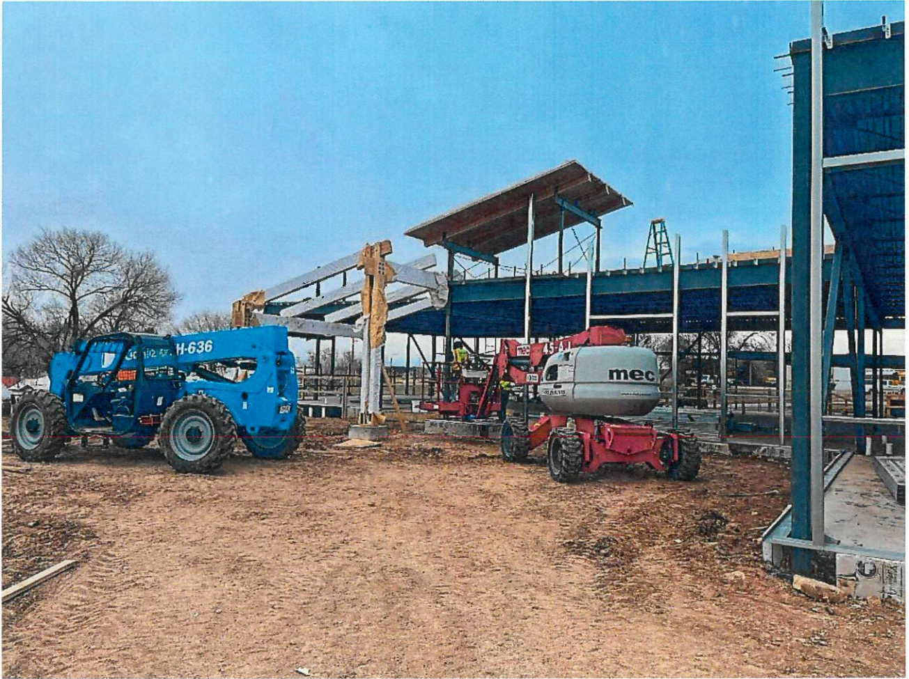
Installation of the glulam beams and wood tongue & groove decking at the main entrance.
