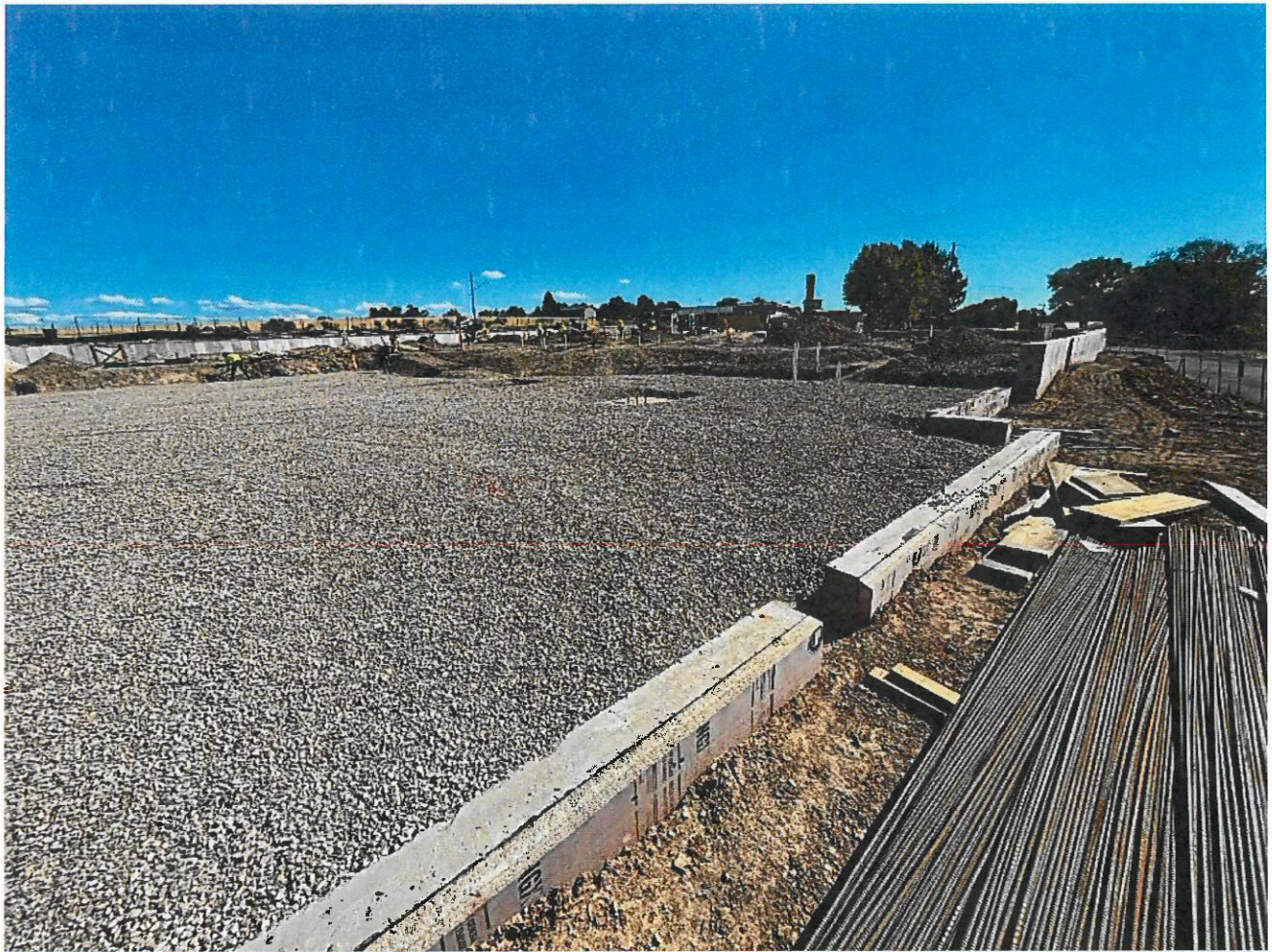
The gym area ready for vapor barrier and rebar to be installed before the slab on grade pour.
