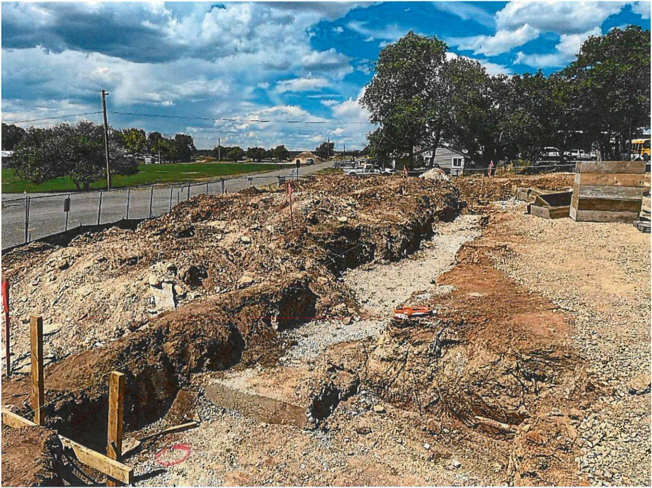
Flowfill has been placed to establish subgrade for the perimeter spread footings along the west end of the site.
